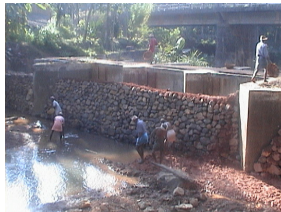
Fig. 5 – An abandoned permanent check-dam due to technical failure while a temporary one constructed in front of it in the Kumbadaje panchayat.
